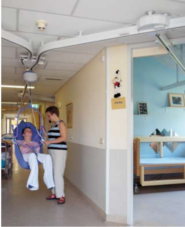
The exchanger and turntable enable a variety of different track solutions.
